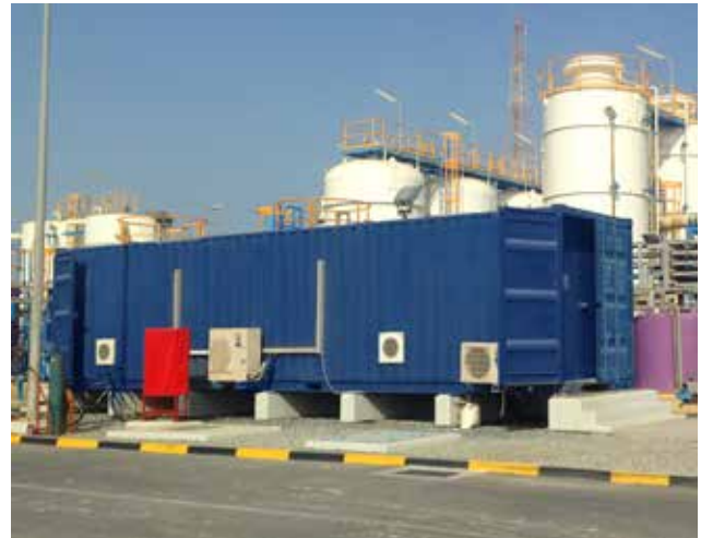
Scotmas Bravo Ultra-Pure duty/standby system in 40' container, installed in desalination plant in Saudi Arabia.
