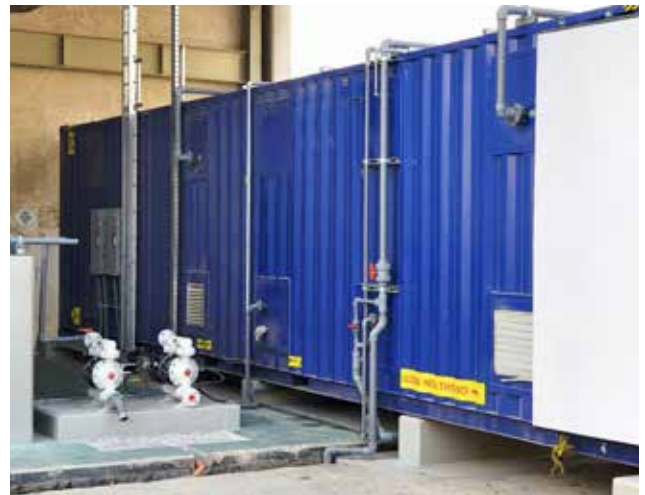
Scotmas Bravo Ultra-Pure duty/standby system in 40' container, installed in desalination plant in Saudi Arabia.
